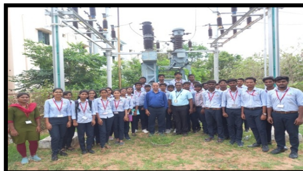
III B.Tech., II sem. EEE, Participant to field Visit to 33/11kV substation, A.rangam Pet, Chndragiri, Tirupathi Andhra Pradesh
