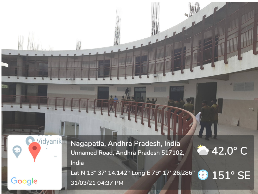
Photographs at Construction Site of New Academic Block G+8 Floors, SVEC Campus
