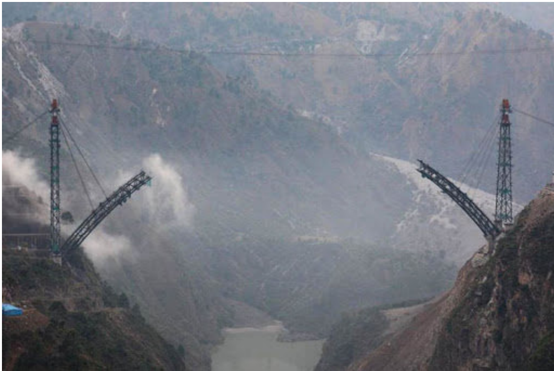
Photograph of World's Highest Railway Bridge - Chenab Railway Bridge Construction as part of presentation
