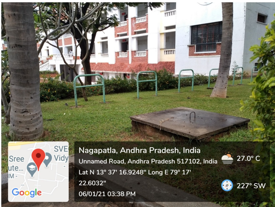
Rain Water Collection and Conveyance System at MNS-Block
