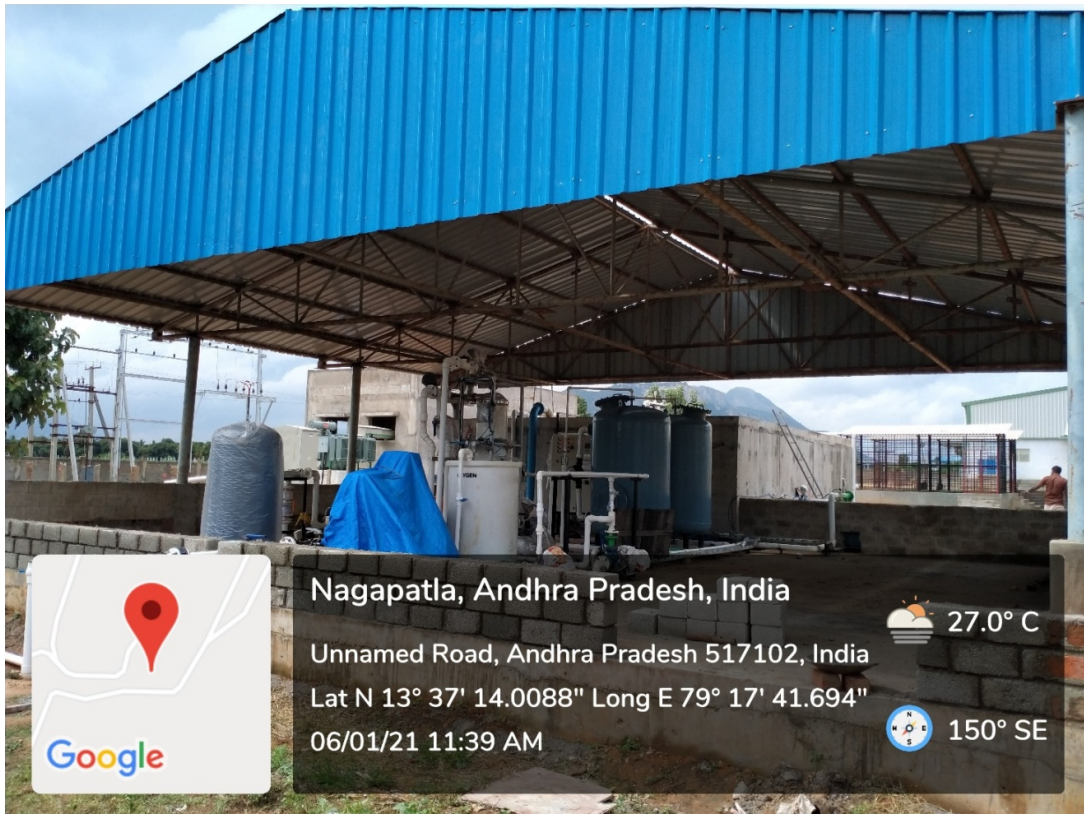
Sewage Treatment Plant of 250 KLD Capacity at V Block
