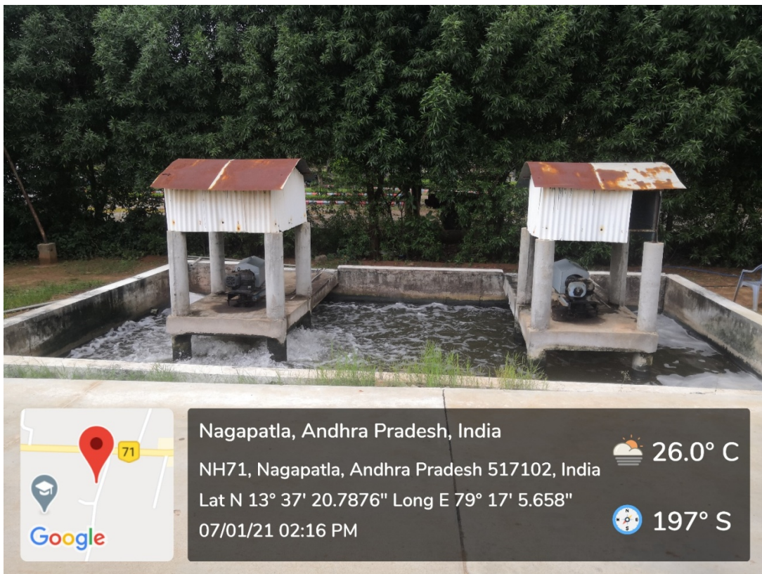
Sewage Treatment Plant of 150 KLD Capacity at Girls Hostels
