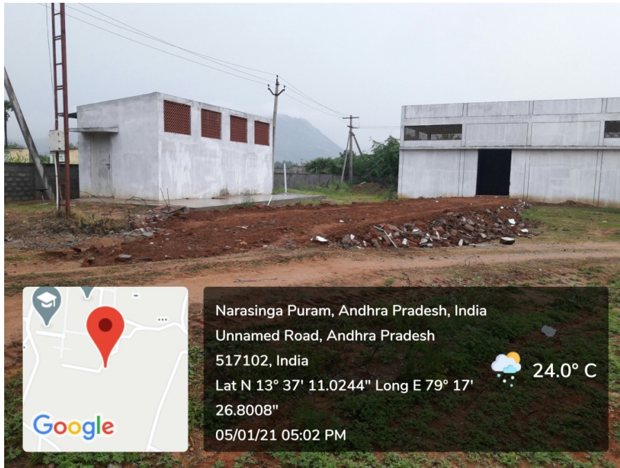
Filling up of Low Lying Area for providing Path for the Toilet Building and Storage Room
