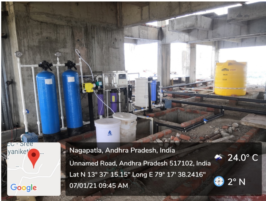
Reverse Osmosis (RO) System (2000 Liters per Hour Capacity) at College Premises
