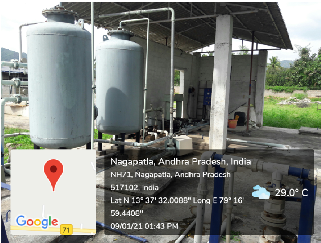
Sewage Treatment Plant of 200 KLD Capacity at Boys Hostels
