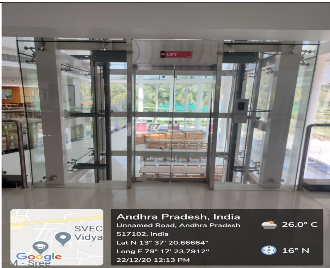
Lift Facility at Central Library
